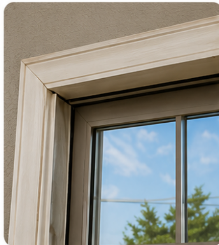
Gaps Around Windows
