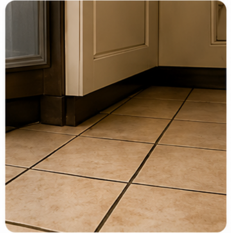
Uneven or Sloping Floors
