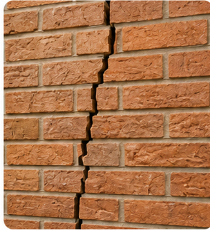
Exterior Brick Cracks
