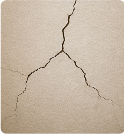
Interior Wall Cracks
