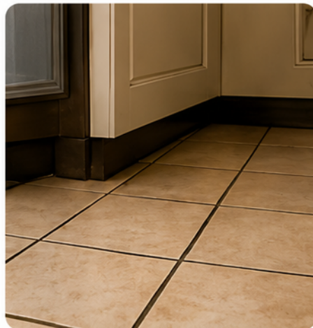
Uneven or Sloping Floors
