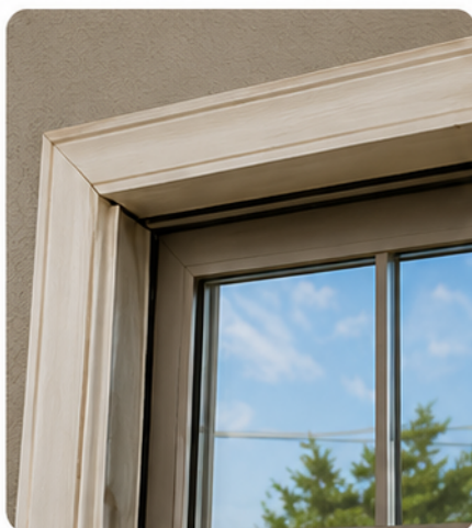
Gaps Around Windows
