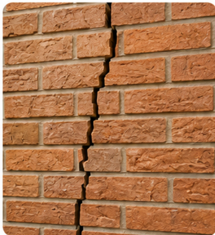
Exterior Brick Cracks
