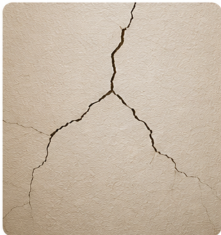
Interior Wall Cracks
